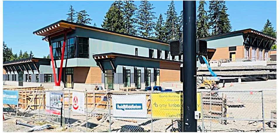
The new Station 111/Headquarters is nearing completion with an anticipated opening this fall.
