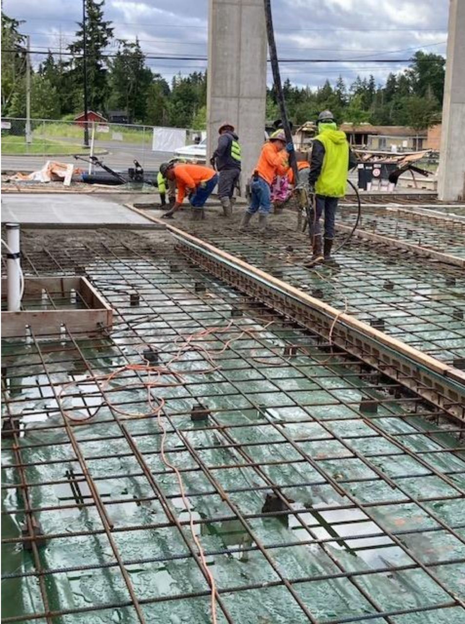
Apparatus bay floor concrete was a two day pour. 90 cubic yards on the first day.
